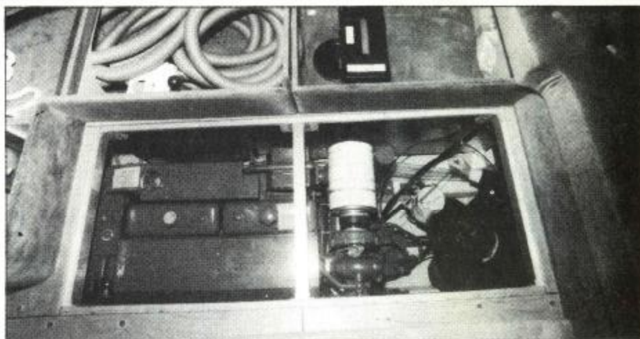
Access to the after end of the engineroom is more easily gained by lifting the hatches in the saloon sole than by working through from forward. The hand bilge pump is back-up for three electric pumps.
